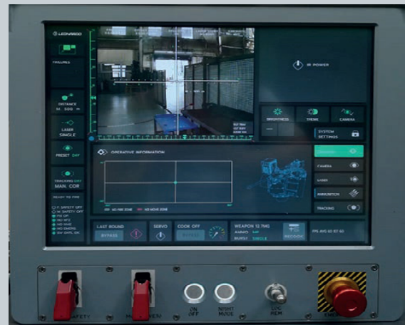
Local Control Panel
